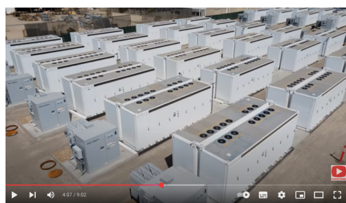
Disaster at Moss Landing: The Risk of Battery Storage
