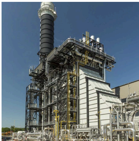
Heat Recovery Steam Generator
